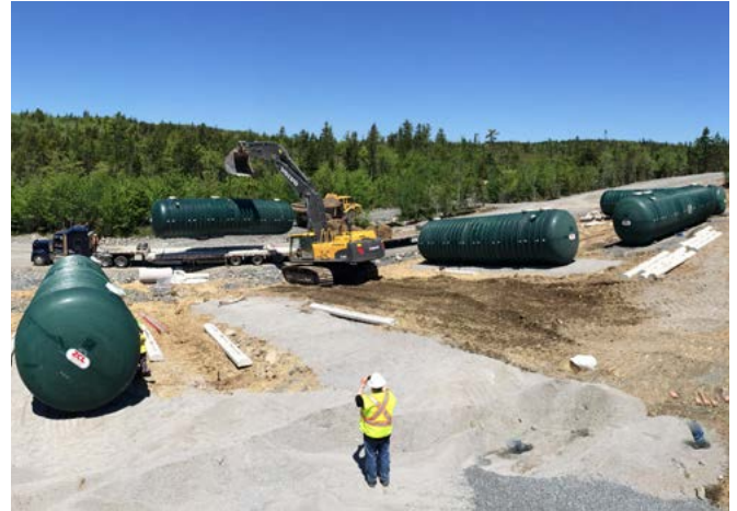
The area consists of lots of bedrock. Gravity sewers would have required large, deep trenches whereas pressure sewer mains are installed just below the frost line.
